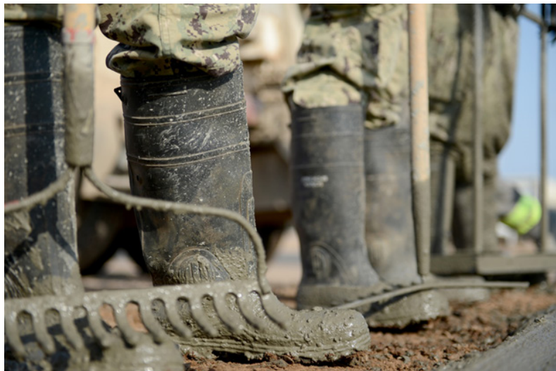
U.S. Sailors assigned to Naval Mobile Construction Battalion 11 pour concrete for a project at Camp Lemonnier, Djibouti.
