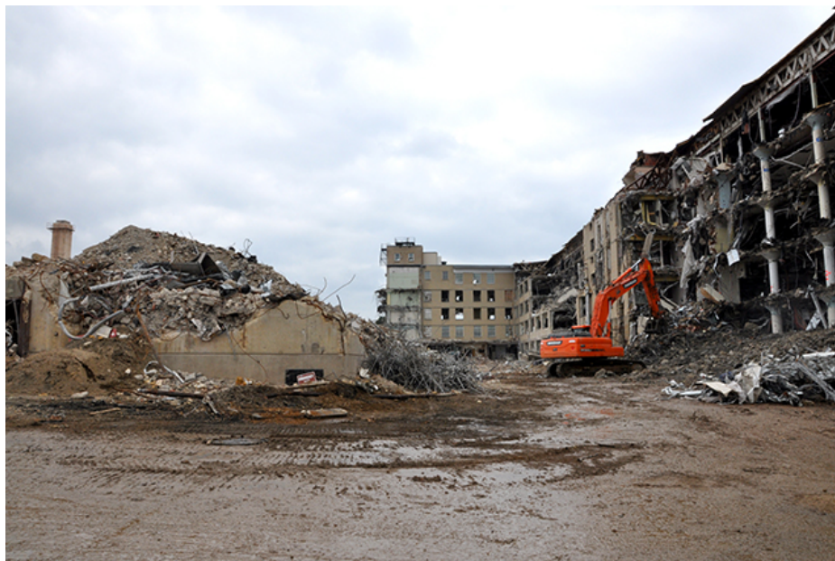
Demolition of the Navy Annex in Arlington, Virginia, began in November 2012. The above picture shows sections of Wing 6 and 7.
