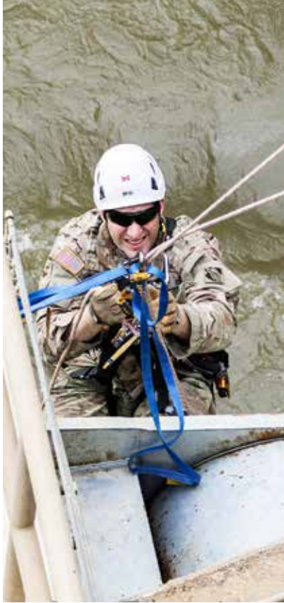
An engineer inspects the gates on a lock and dam. (U.S. Army Corps of Engineers photo by Thomas Mills)
