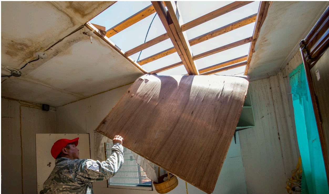
U.S. Air Force Tech. Sgt. Frank Babauta, a structural craftsman with the 254th Rapid Engineer Deployable Heavy Operational Repair Squadron Engineers, assesses a home damaged by Super Typhoon Yutu in the village of Koblerville, Saipan, Commonwealth of Northern Mariana Islands, Nov. 12, 2018.
